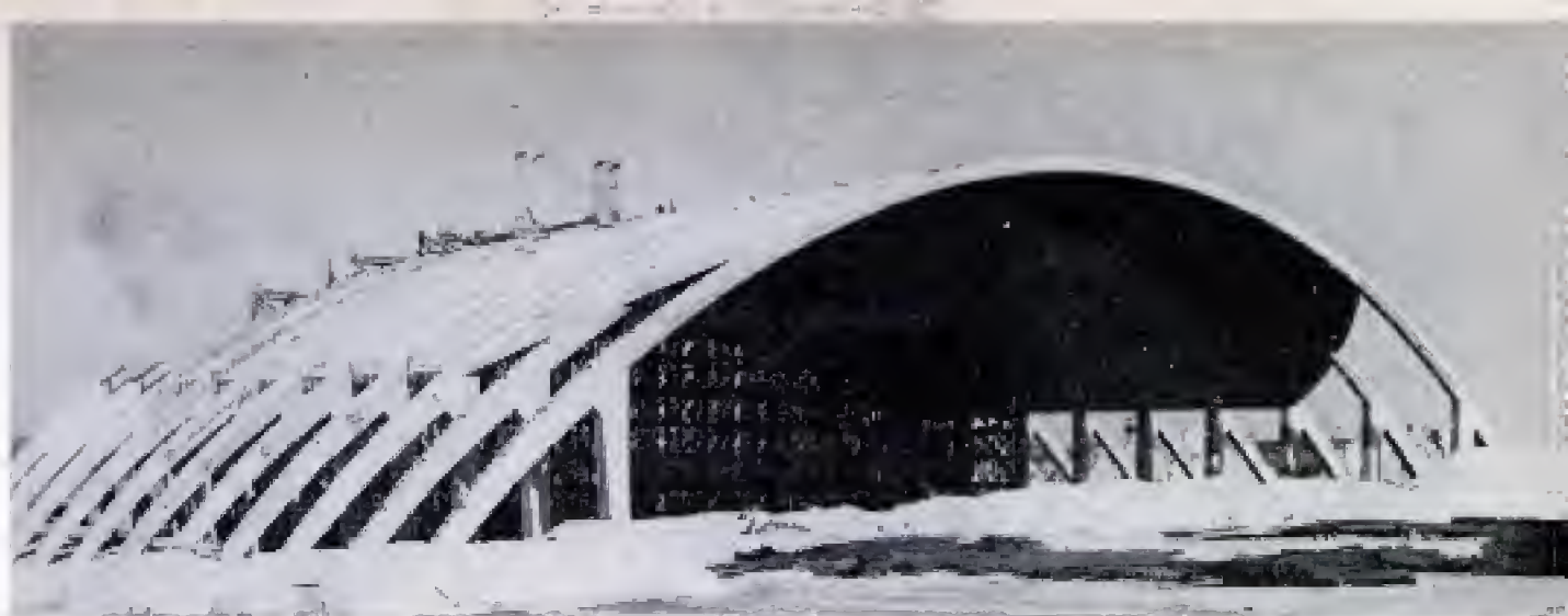
Interior scaffolds moved along on tracks as ribs were mounted and roof was laid. Arches at rear are unfinished
